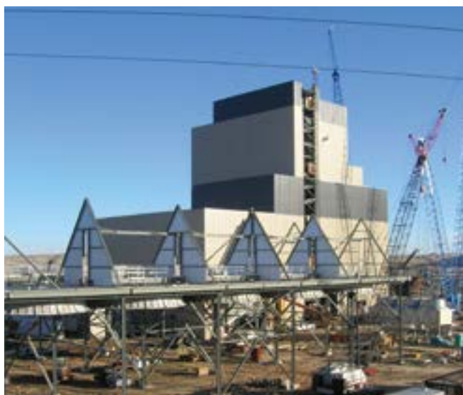
Wygen II under construction in 2006. A 90 MW, coal-fired, base load power plant, Wygen II would serve Cheyenne Light customers. Equipped with mercury scrubbing technology, the plant was intended to be among the cleanest conventional coal-fired plants in the nation.
