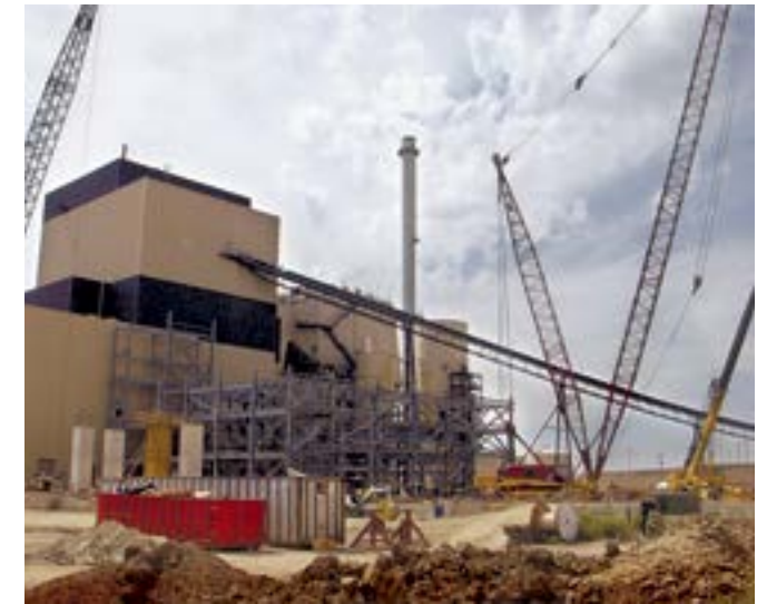
Wygen I under construction in 2002. One of the cleanest coal-fired power plants in the U.S., Wygen I was nominated for an EPA Clean Air Award after it went online in 2003.
